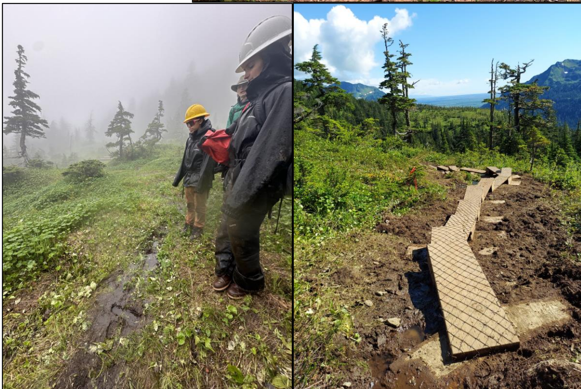
Pictured Above: Step-n-Run Construction Before (left) and After (right) on the Mike O'Leary intertie trail.
