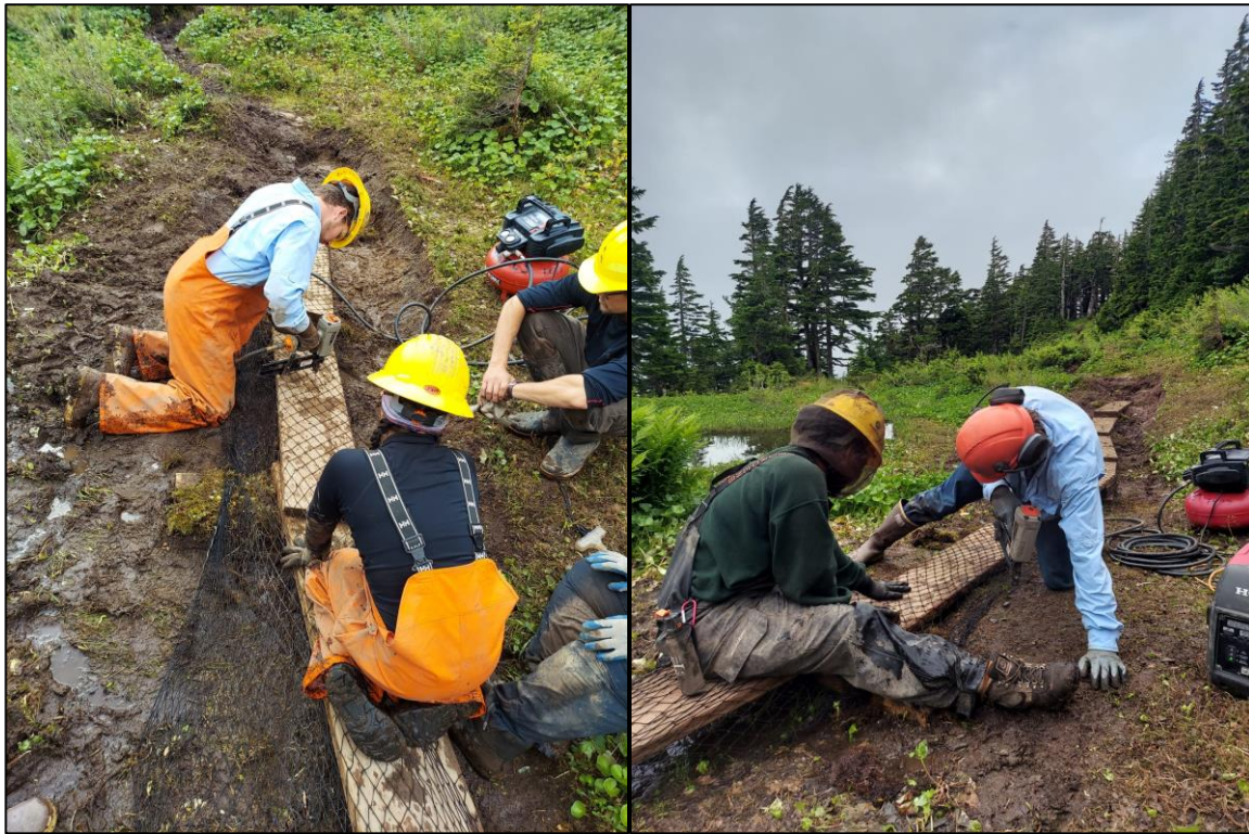
Pictured Above: Crew Members Installing netting on the Step-n-Run Construction with Staple Gun.
