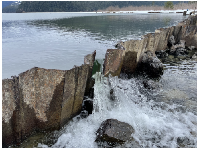
FIGURE: Sheet Pile Joint Burst
