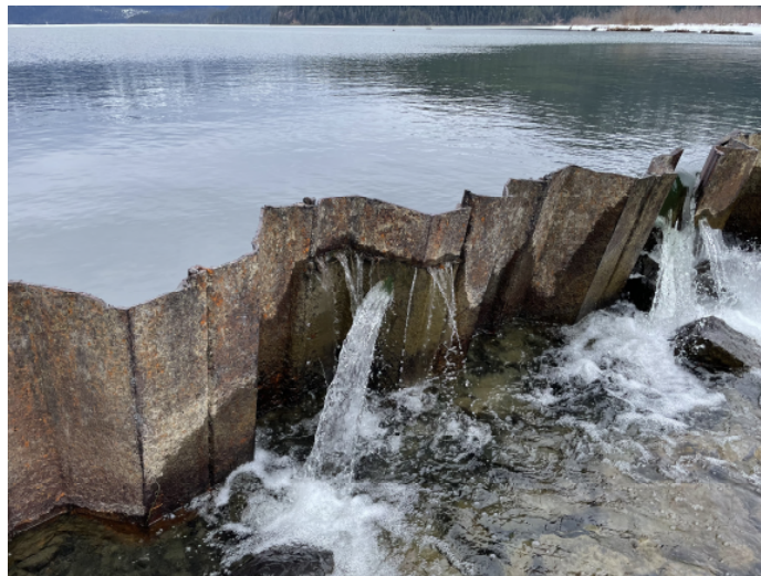
FIGURE: Material Degradation and Leaking
