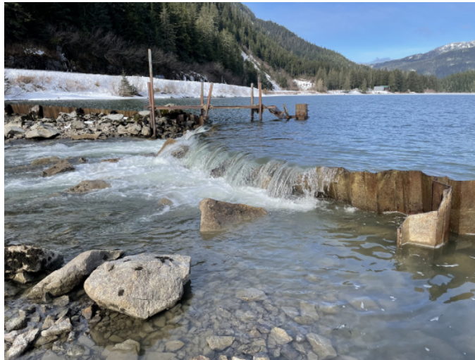
FIGURE: Sheet Pile Failure Lowering Crest of Weir
