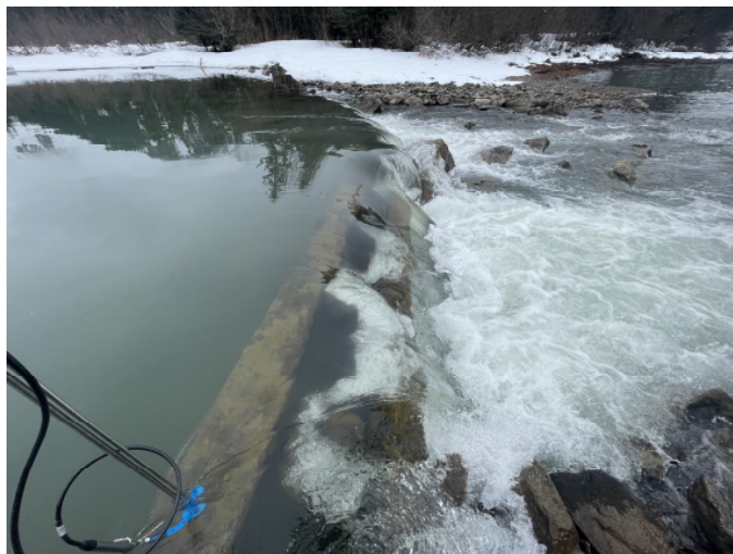
FIGURE: Failed Section of Crest
