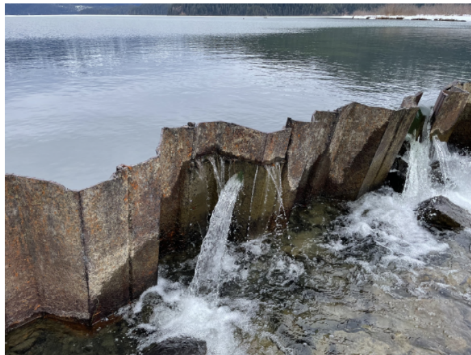
FIGURE: Material Degradation and Leaking
