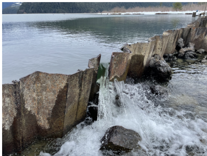
FIGURE: Sheet Pile Joint Burst
