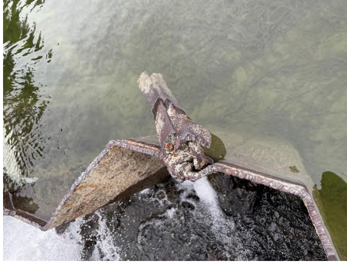
FIGURE: Leaking of Sheet Pile Joints
