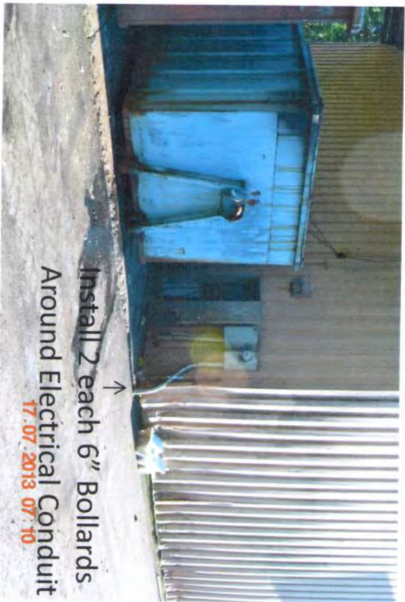
East Face - Electrical Service (N.E. Corner of Building)
