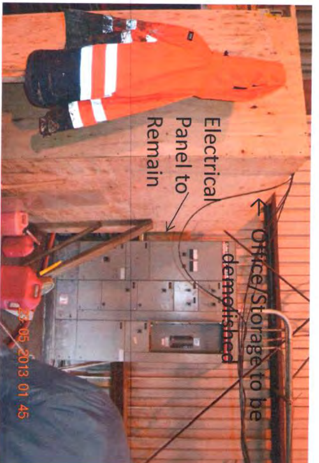
Electrical Panel Northeast Wall
