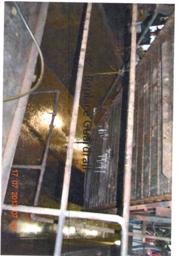
East End - Pit Under Baler Machine
