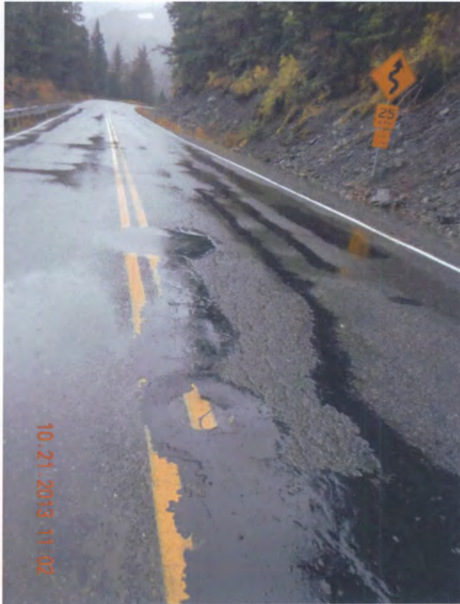
Figure 2. Site photo of road damage and sloughed material in the ditch line.
